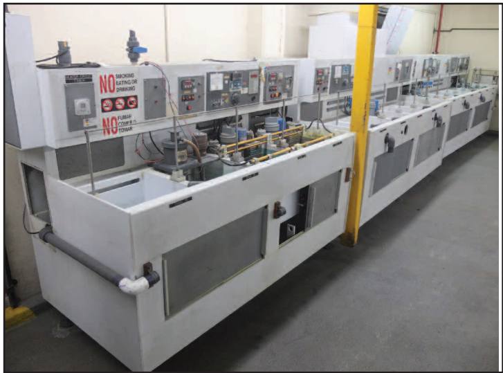
PLATING TANK LINE
