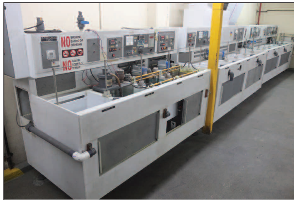
PLATING TANK LINE
